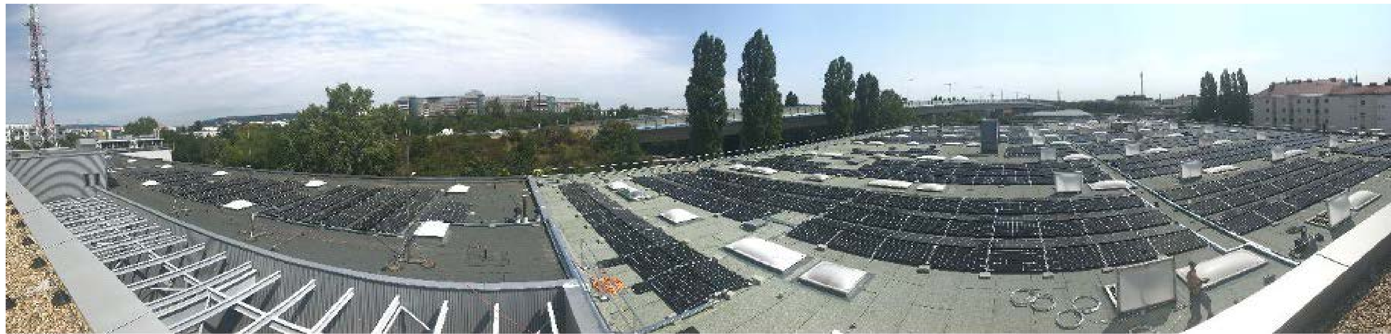
ON-SITE SOLAR AT 3 AUSTRIA
