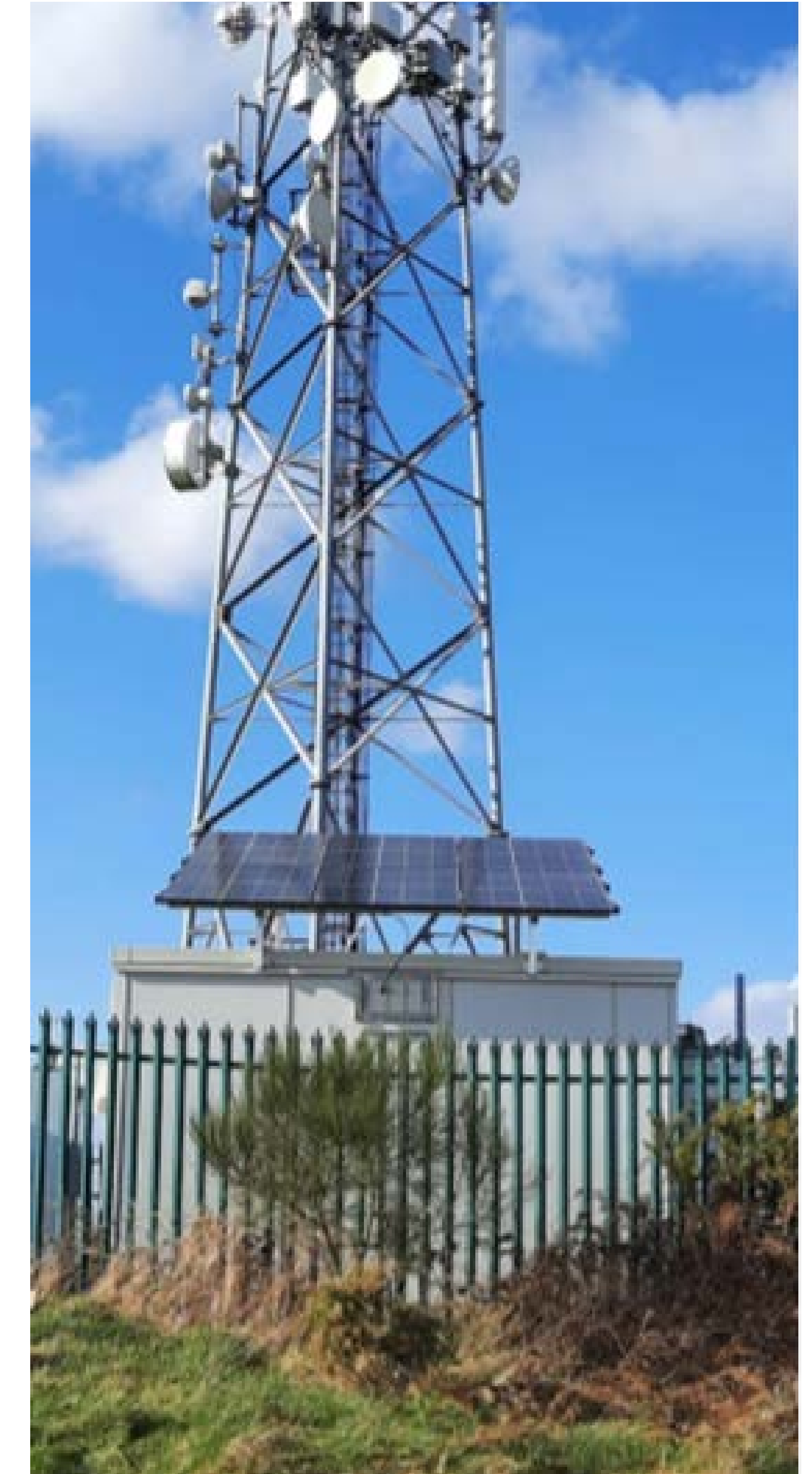
ON-SITE SOLAR GENERATION AT 3 IRELAND
